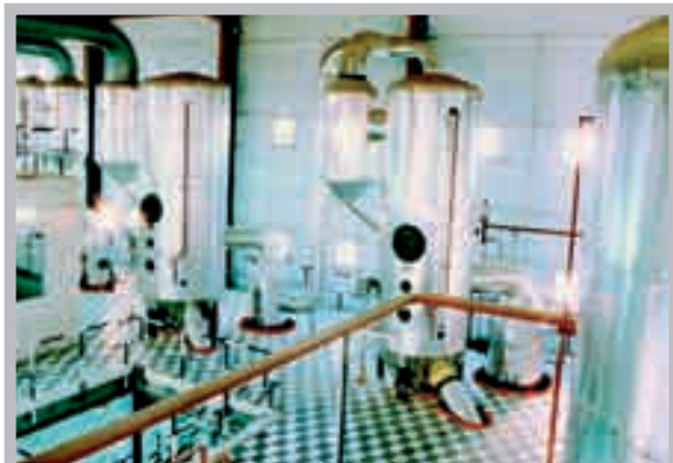
Sweet waters evaporation plant - Capacity: 100 t/d
