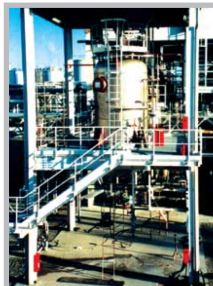
"Dead-End" type fatty acids hydrogenation plant Capacity: 16 t/batch
