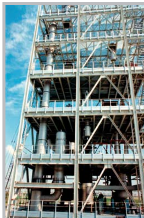
Fractionating column and falling film evaporator
