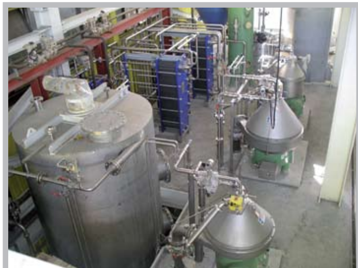
Line of centrifugal separators for neutralizing/degumming plant
