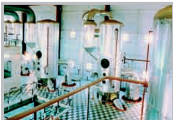
Sweet waters evaporation plant - Capacity: 100 t/d
