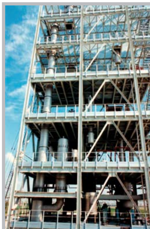
Fractionating column and falling film evaporator
